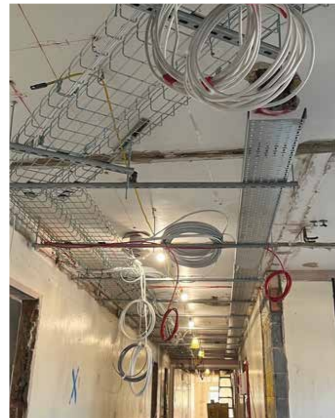
Caption: The electrical cables
