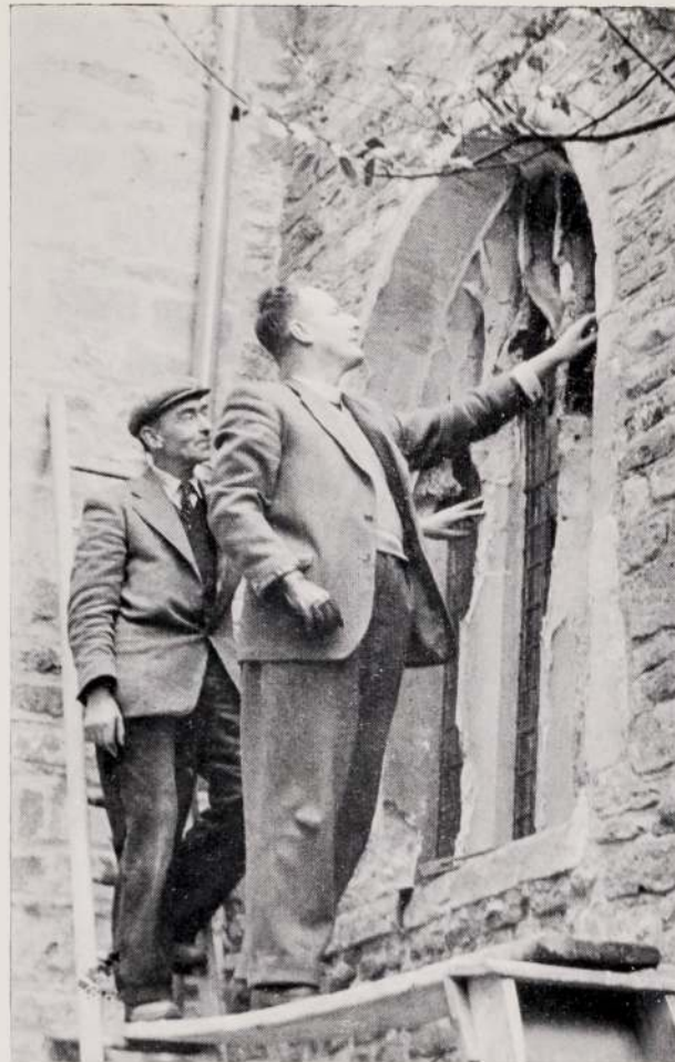
With his builder, Mr. Treglown scales stepladder and board to examine by touch the damage to a window of St. Mary's Church.
