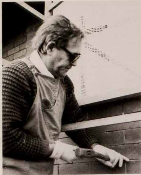
Tony chips out the sand and cement, careful not to chip the brickwork.
