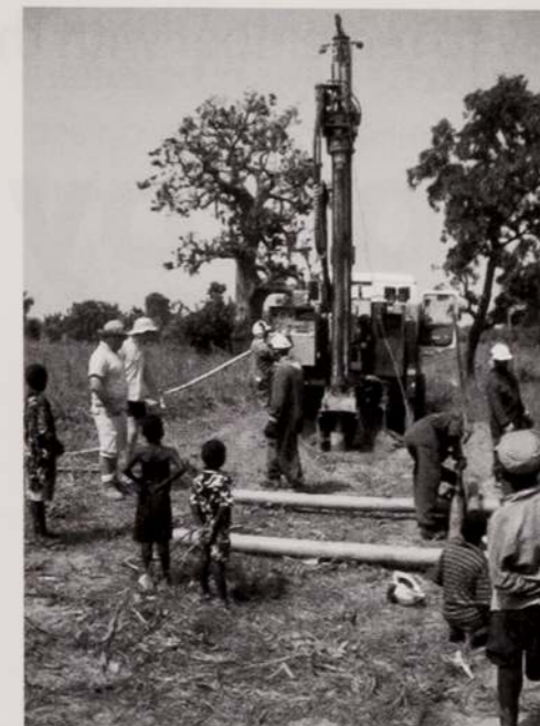
The team drill a borehole though the chances of finding a consistent water supply are slim.
